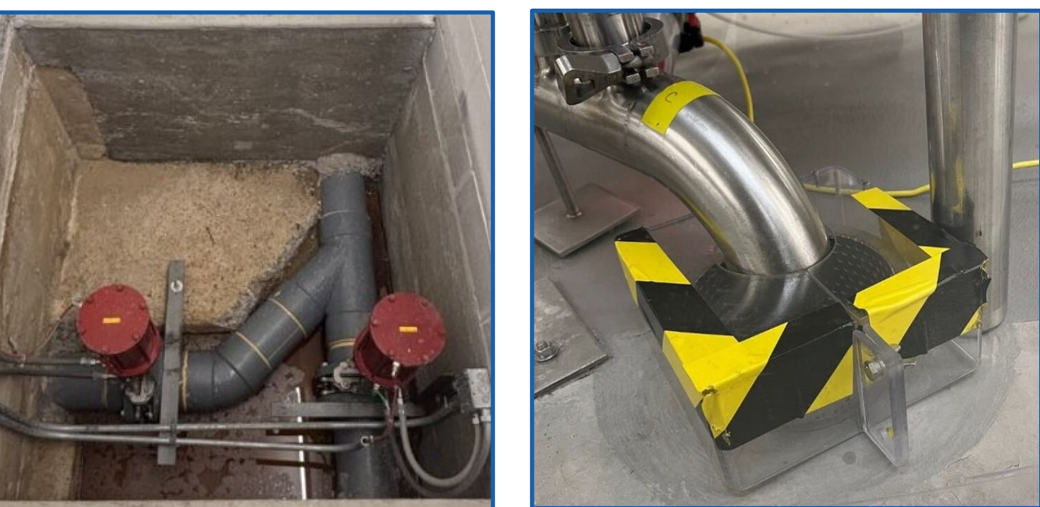
Figure 2. Main wastewater pipeline Y-split.
