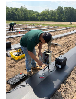
Fig. 2. Sensors installed in plots
