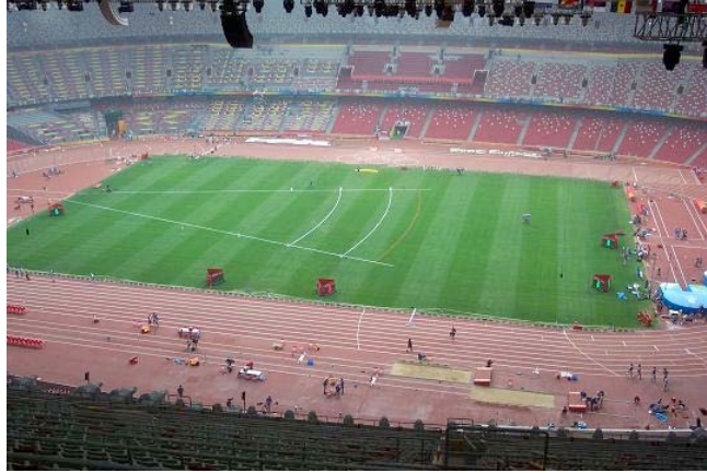
Image 5: Modular field after its installation prior to the initiation of track and field competition, August 13, 2008, National Stadium, Beijing, China.
