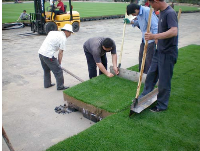
Image 1: China Sports Industry Group Co. moving established GreenTech® ITM™ modules at the modular field construction site located on the outskirts of Beijing, China, May 8, 2008.
