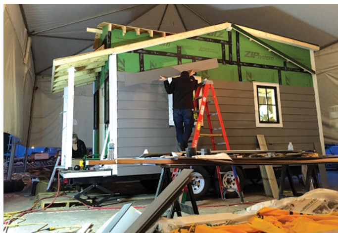
In true LA fashion, an all-night work crew to get the interior and exterior wall coverings installed for the ribbon cutting.
